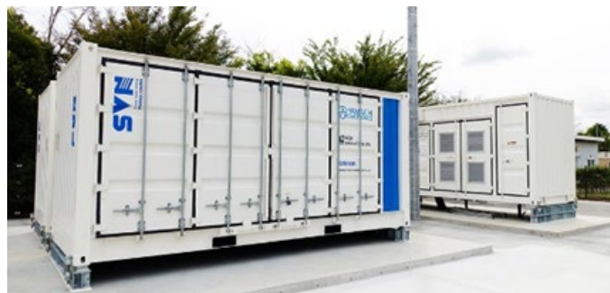
Sakura Factory NAS battery system
